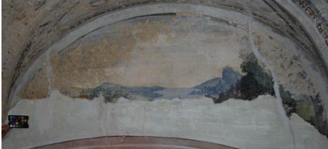
Fig 24 - Thick multiple layers of whitewash on the South-East wall above the entrance to the Chapel
