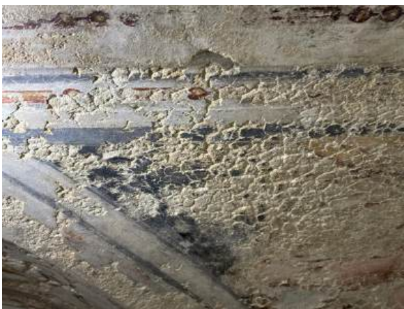
Fig 34 - Shrinkage cracks and material loss.
