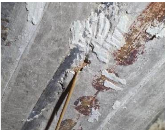
Fig 11 - Loss in plaster layer with view of brick of the support
