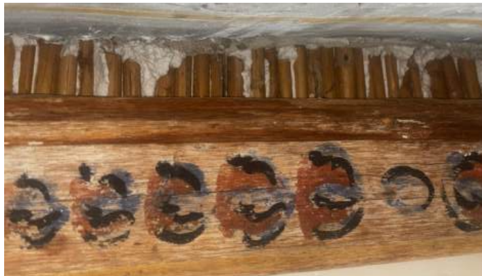
Fig.17 Traces of deterioration of wood
