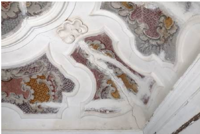
Fig. 14. Visible localised fissures and cracks
