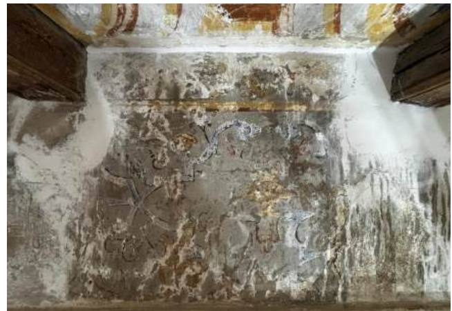
Fig.15. Salt Efflorescence and dampening
