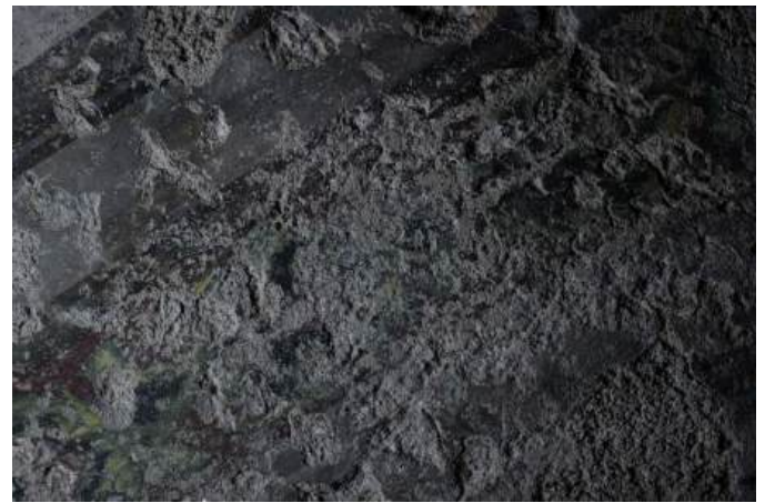
Fig.68. Deposition of dust, discoloration due to deposit
