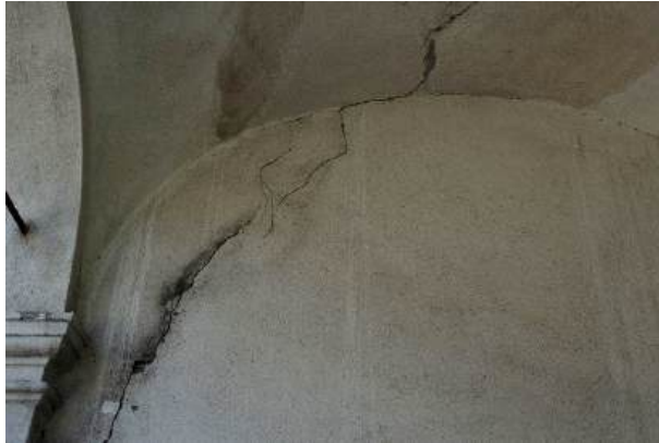
Through crack, exterior
