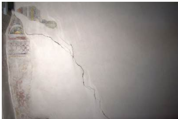
Fig.62. Fissure in the adjacent west wall
