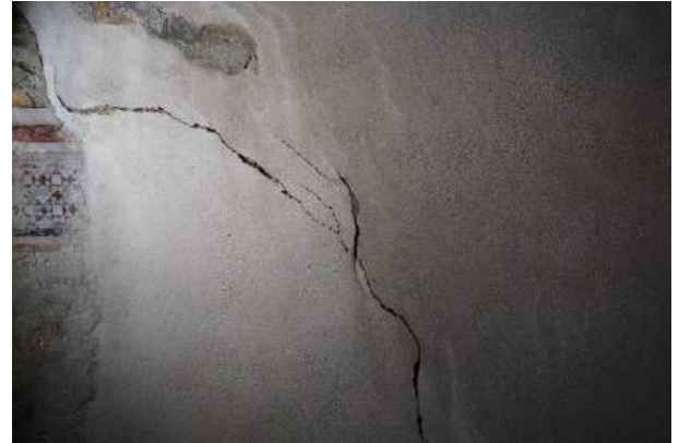
Through crack, interior
