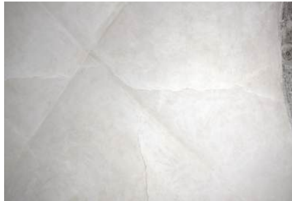
Fig.64. Cracks in the ceiling
