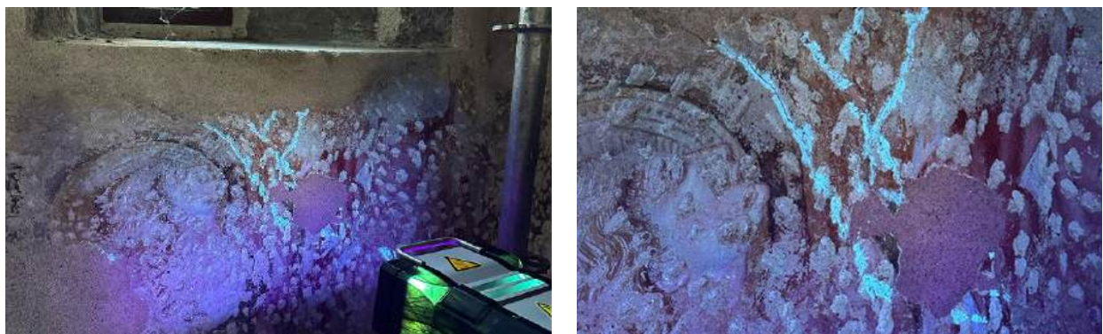
Fig.60,61. Luminescence detected in the fillings under the window
